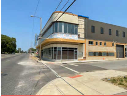
The Mickey's building at Euclid Ave. and Woodlawn Ave. during the renovation process.
